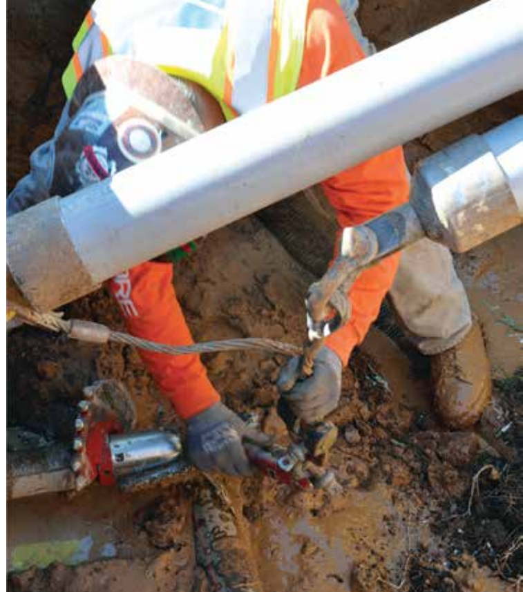
Attaching cable and product to the swivel in preparation for a direct pullback with the FastBack System. The cutter on the FastReam housing will enlarge the bore to pull multiple pipe
